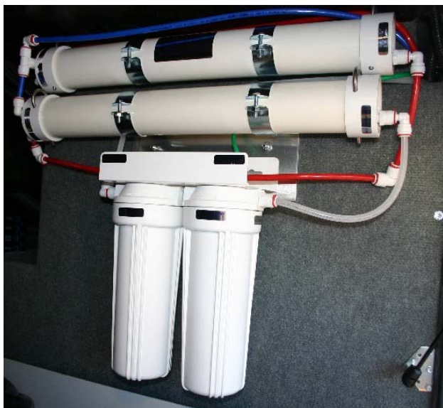
DOUBLE MEMBRANE SYSTEM INSTALLED IN THE TRAVEL SUPREME TWO MEMBRANES DOUBLE PRODUCTION WITHOUT AN INCREASE OF WASTE WATER
