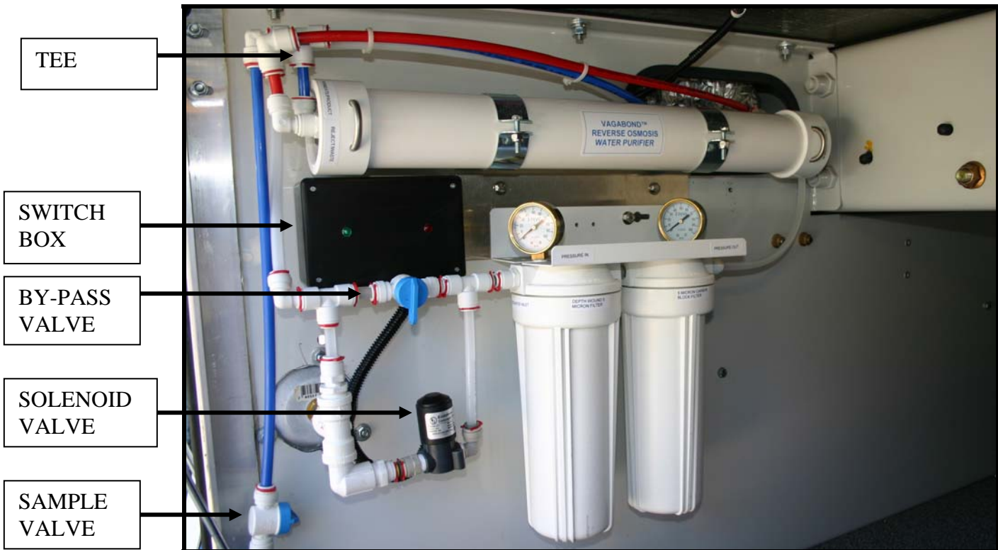
PHOTO OF FULLY AUTOMATIC INSTALLATION
