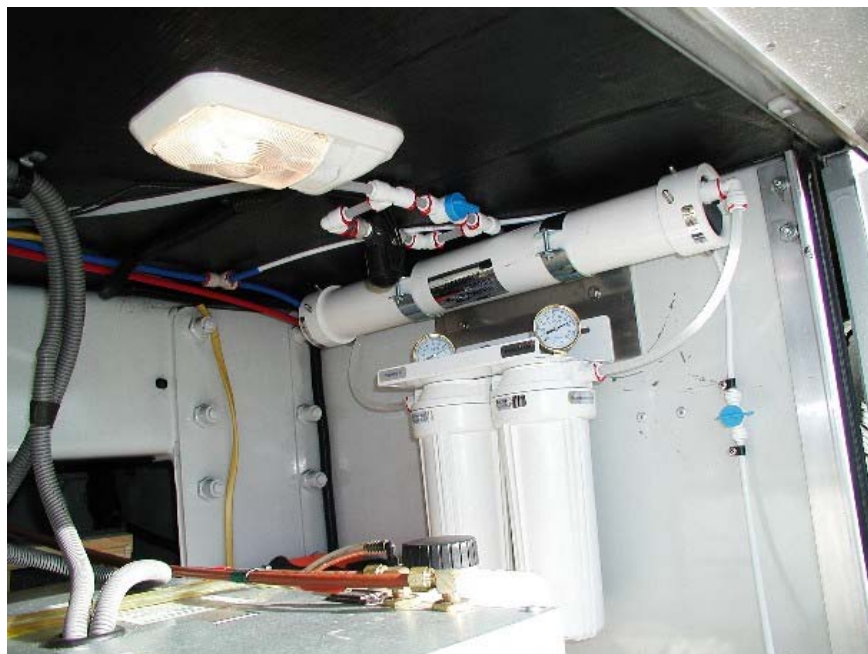
INSTALLATION IN ALPINE HYDROHOT BAY
