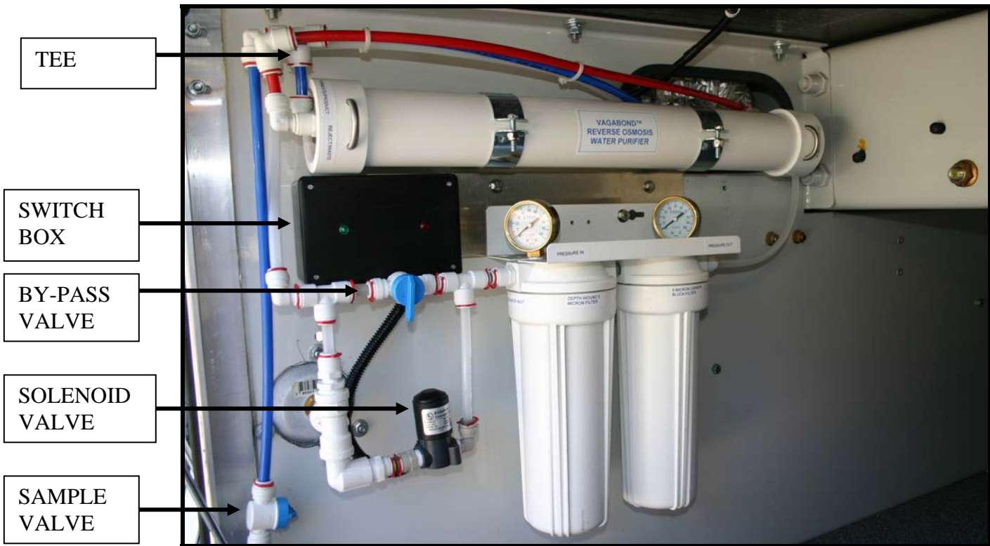
PHOTO OF FULLY AUTOMATIC INSTALLATION
